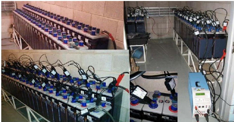
Figure 2: Connection of BVM's and load bank to the battery
